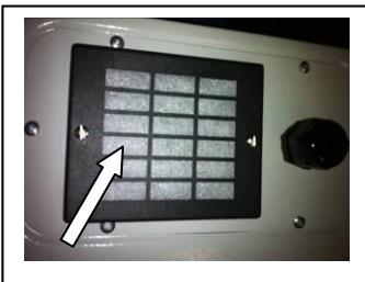
Fig 1 - Electric Panel Filter
